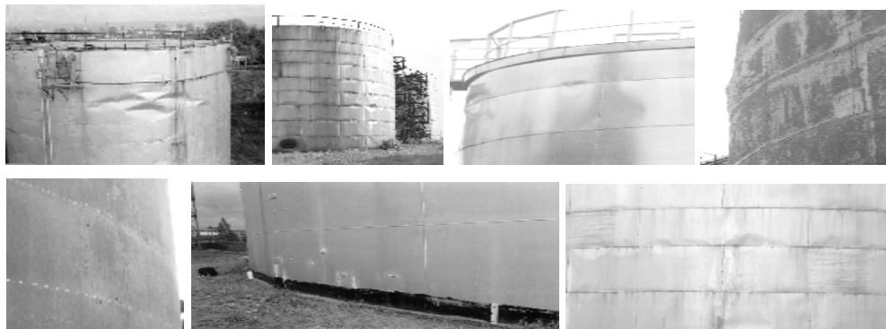
Figure 1: Examples of local shape defects on a wall of steel cylindrical tanks
